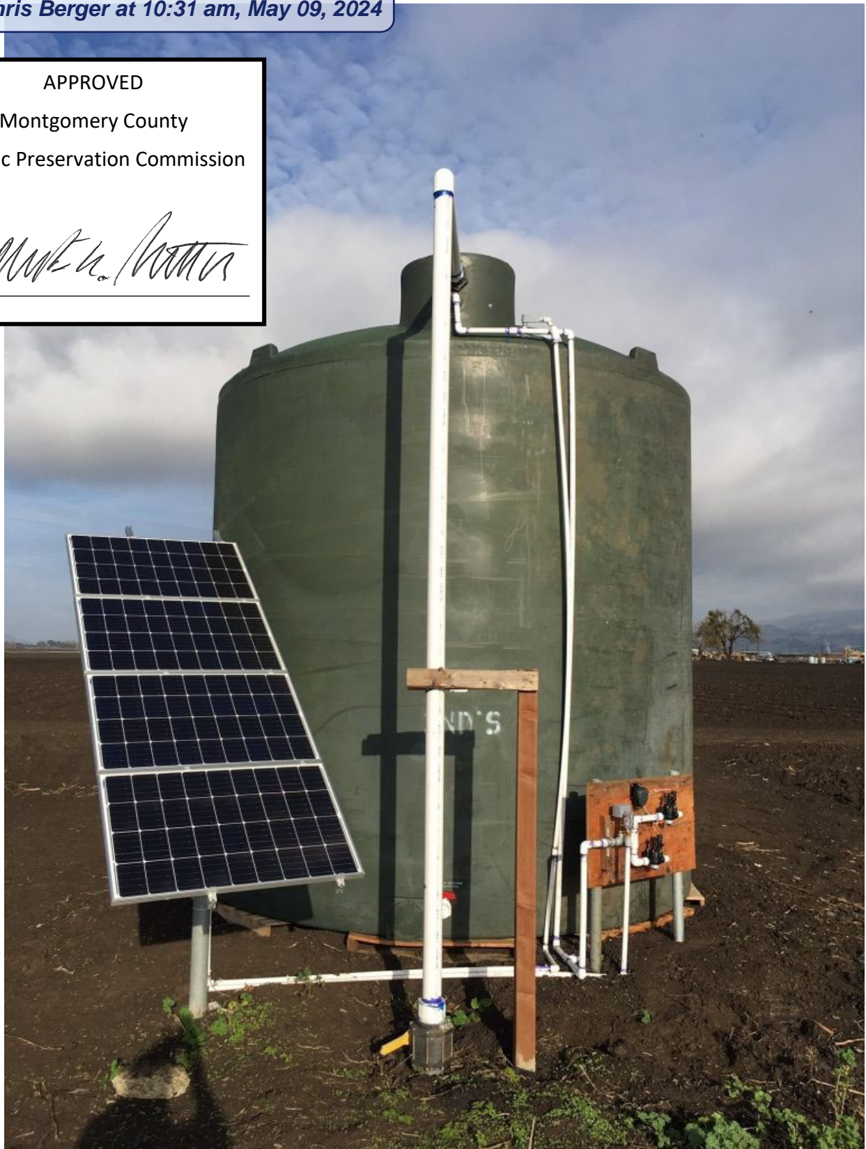
Sample photo of solar charger and above ground plastic water storage tank
