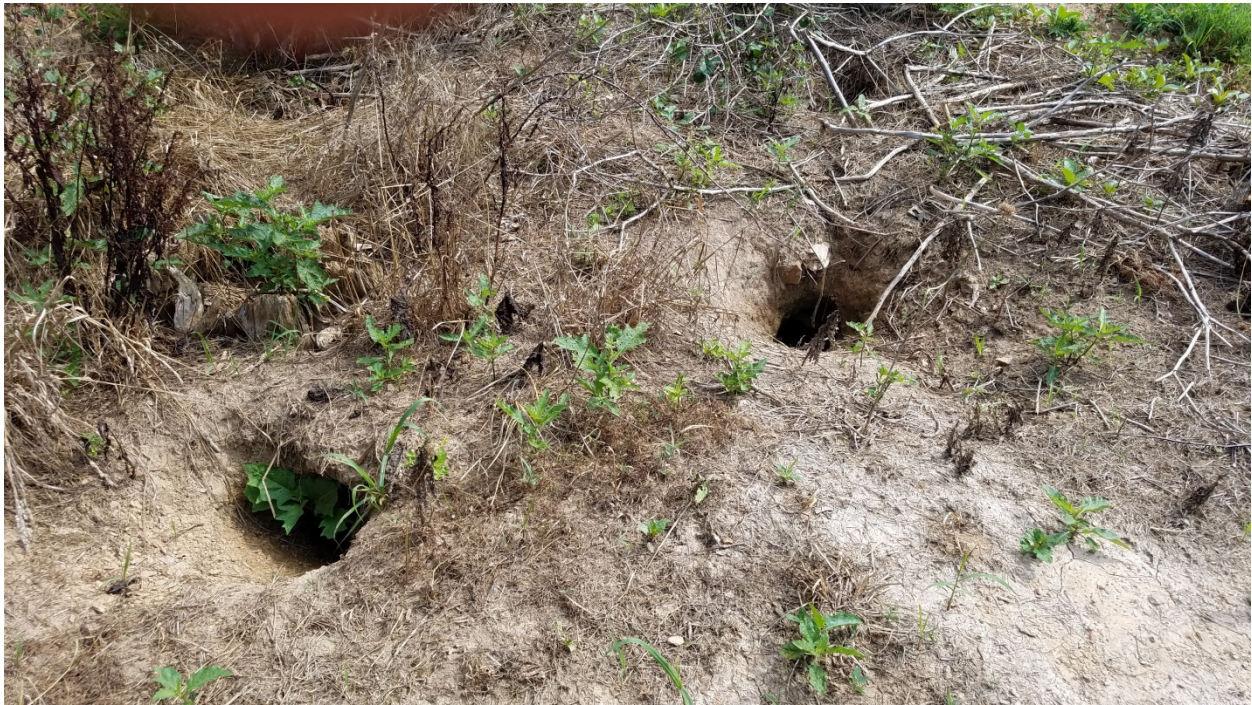
13. Groundhog hole damage throughout cemetery
