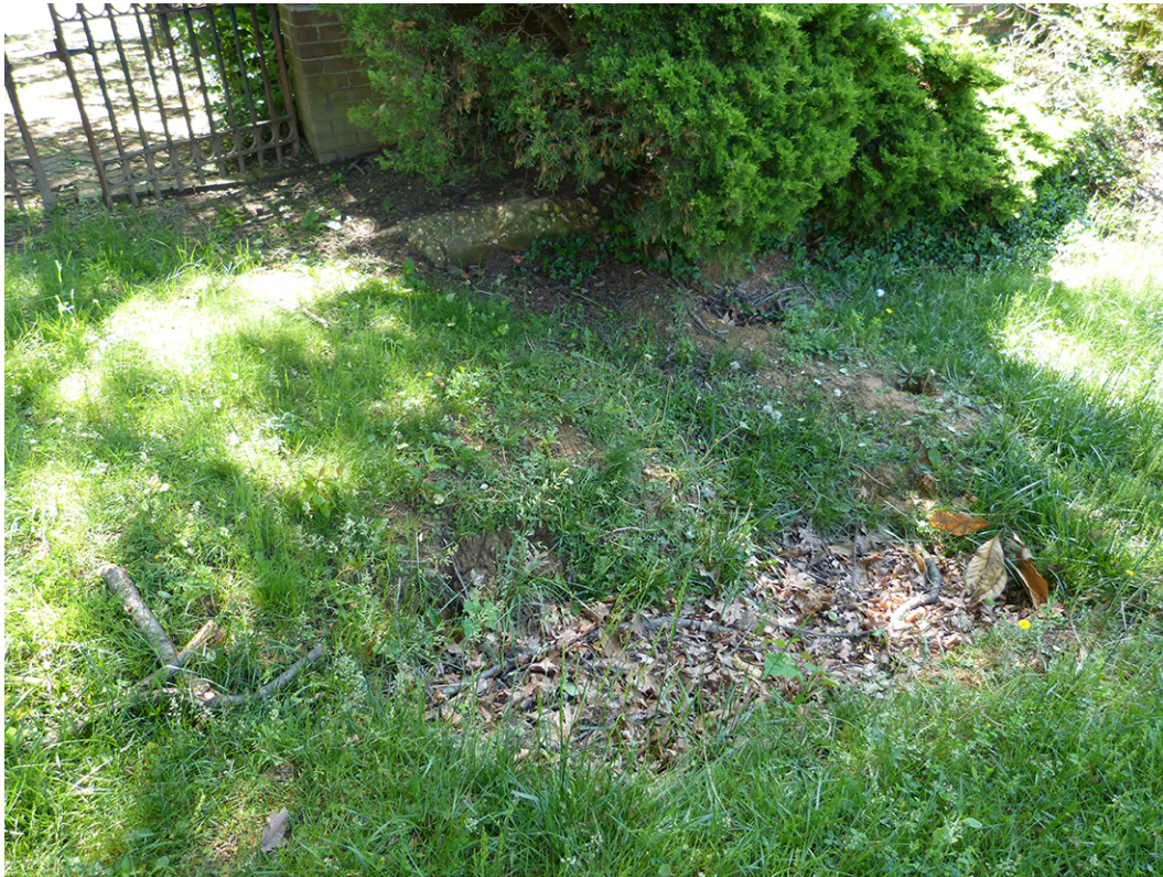
4. Concrete ledge and large depression inside gate
