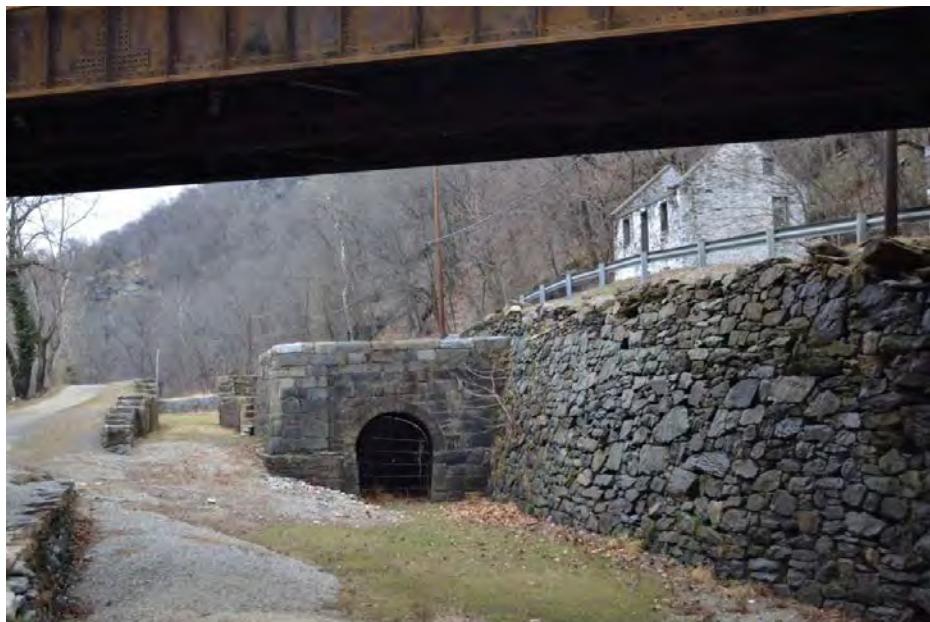
Photo #19 - Mile 60.62A, 60.62B, 60.62 (Map 12). View NW to Lock 33 (11808), Bypass Flume Lock 33 (11809), and Maryland Heights, Bldg. #80, Stone House (45430) in Sandy Hook, MD. (Railroad overpass in this image is not part of the C&O resource inventory.)
