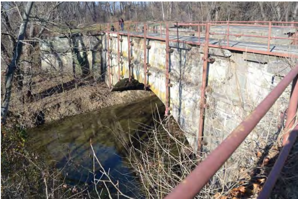
Photo #43 - Mile 180.66 (Map 29). View NW to stabilized Evitts Creek Aqueduct (12855), south of Cumberland, MD
