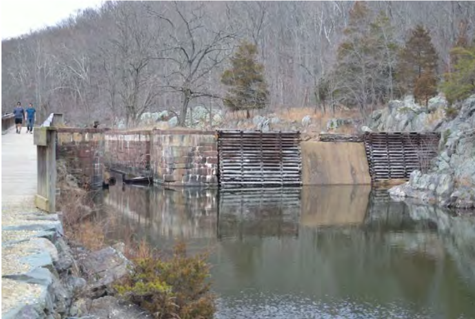
Photo #8 - Mile 13.45, 13.45A (Map 3). View N to Lock 15 (12721) shows Seneca red sandstone construction (1830), wooden cribs (1939-1942), and concrete wall (1975); and Bypass Flume – Lock 15 (12722) south of Great Falls, MD
