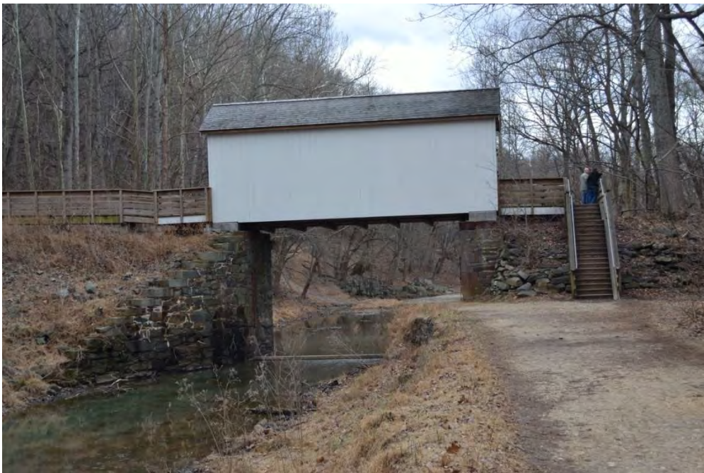
Photo #9 Mile 13.75 (Map 3). View S to Stop Gate (12723) between Locks 16 and 17, with rebuilt bridge and winch house south of Great Falls, MD
