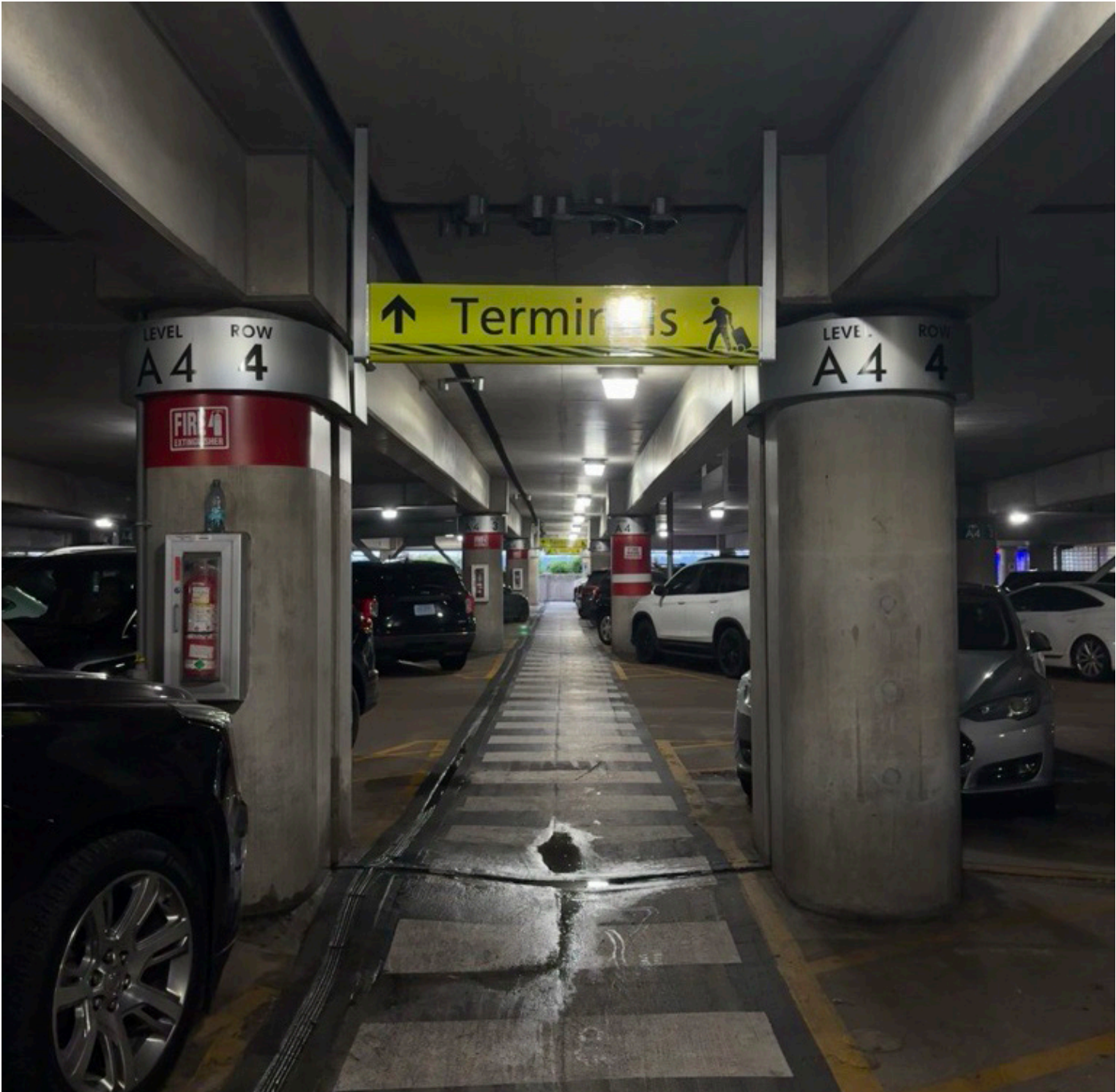
FIGURE 50 Example of insufficient lighting in parking garage impacting feeling of safety
