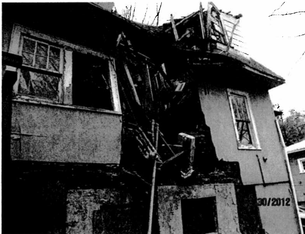
4. Close view of collapsed roof and second floor.
