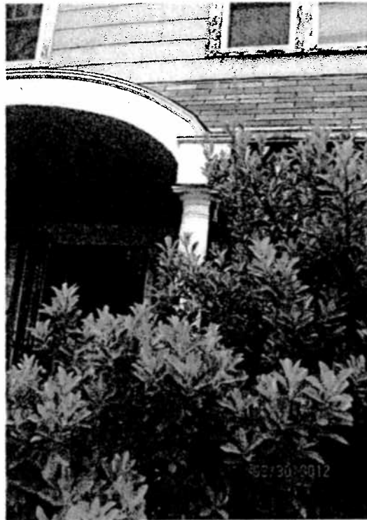
9. Structural damage to front porch structure.
