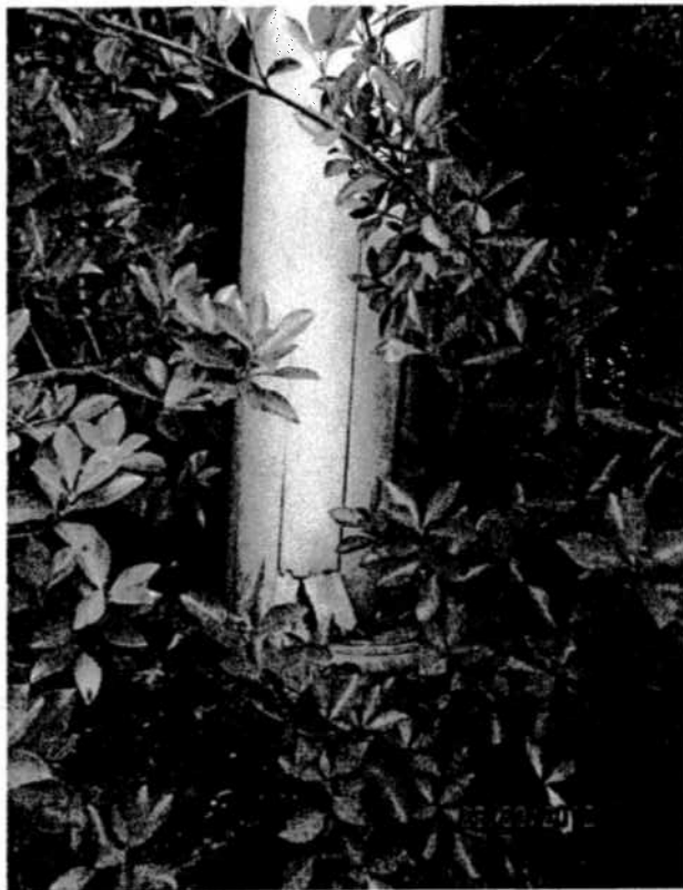
12. Close view of right porch column dislodged from base and column is damaged.
