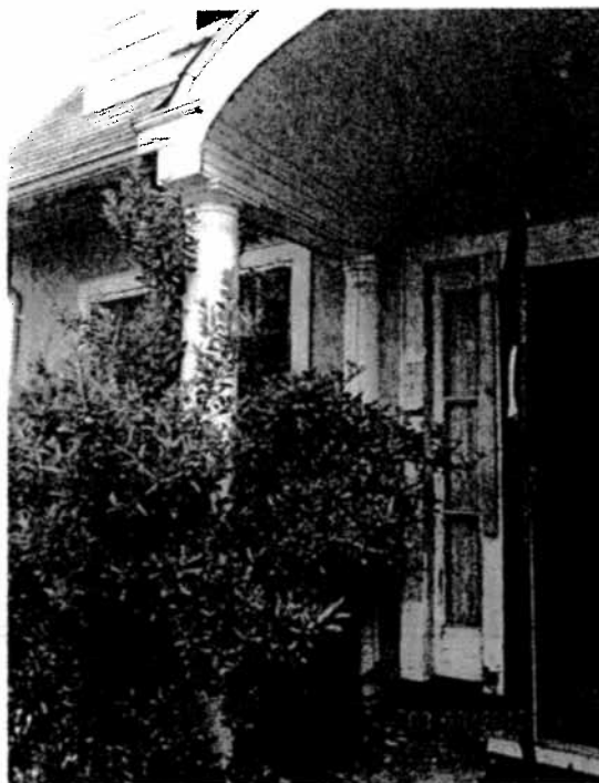
10. Structural damage to front porch structure. Also note termite tubes on rear column.
