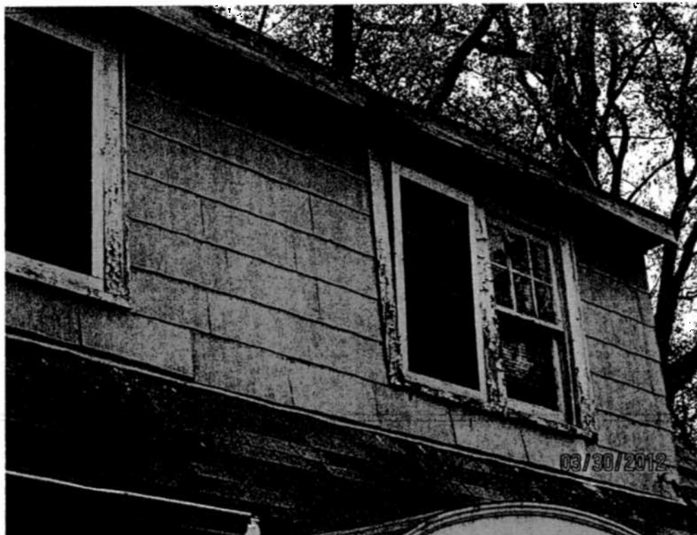
8. Close view of roof rot damage.
