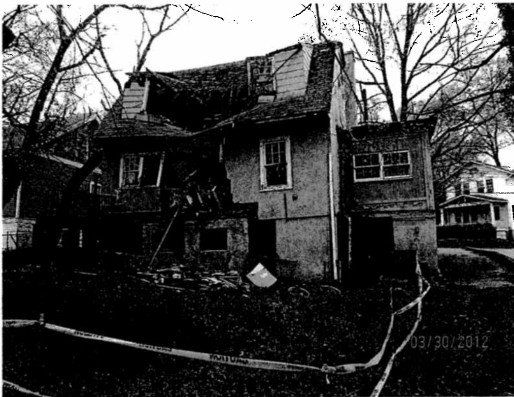
2. Rear view of house showing damage from tree falling onto house
