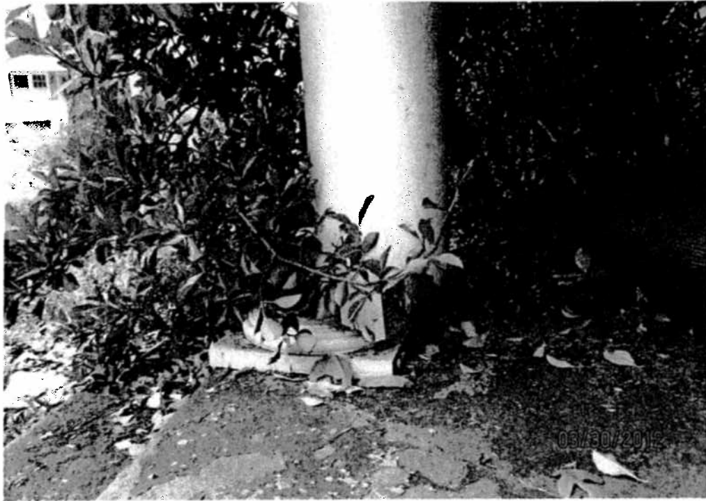
11. Close view of left porch column dislodged from base and column is damaged.
