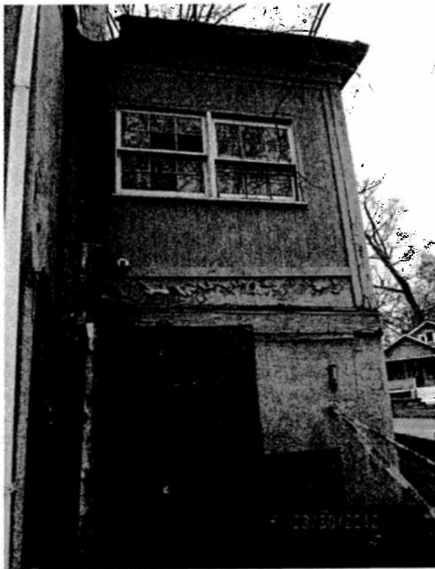
6. Side addition has detached from house.
