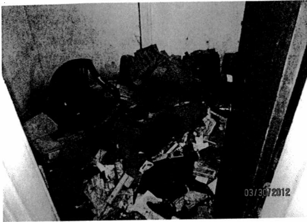
19. Interior view of collapsed first floor on east side of house from wood rot.
