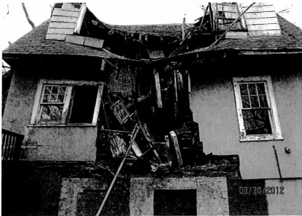
3. Close view of collapsed roof and second floor.
