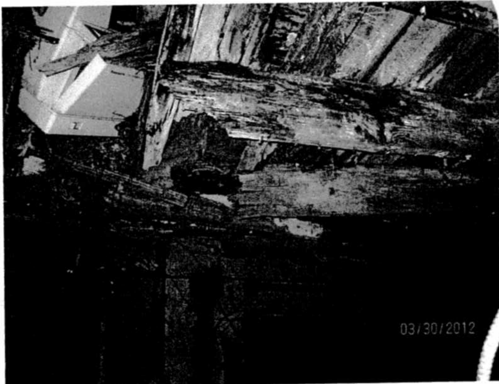
20. Interior view of first floor collapse into basement from wood rot.
