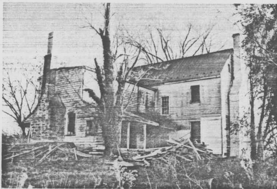
Rear View of Mount Nebo Prior to Restoration
