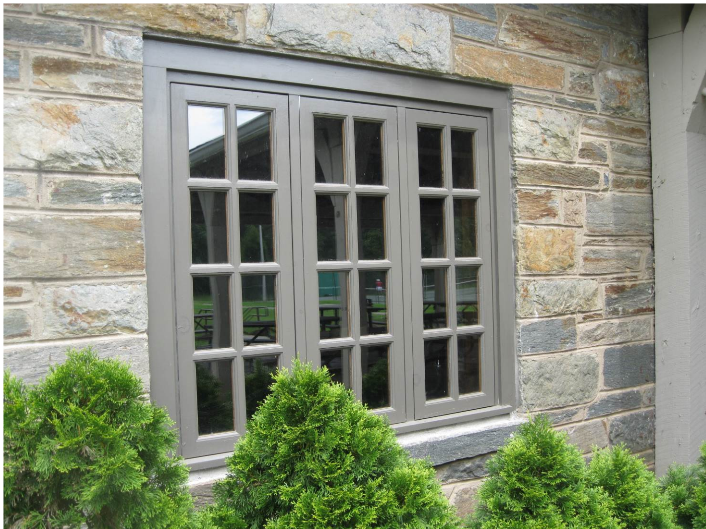
Figure 22. Detail of replacement casement windows, modeled after original windows seen in ca. 1940 photos.
