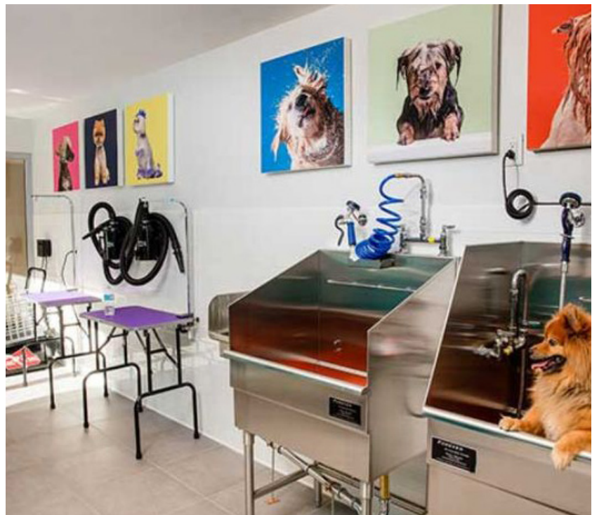
Example of a dog washing facility in a multifamily complex, Greenville, SC
