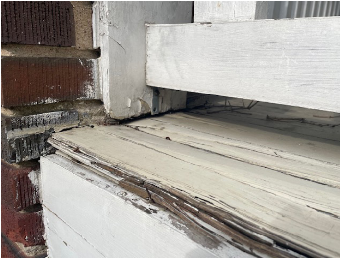
detail of damage at south end
