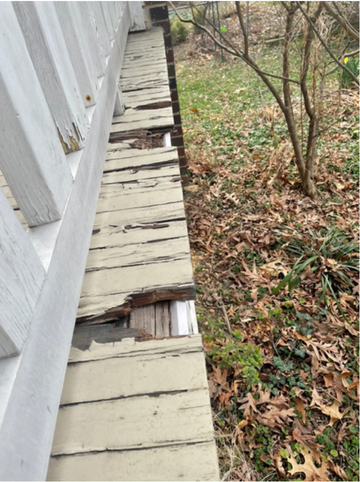
detail of damage at west edge (top)
