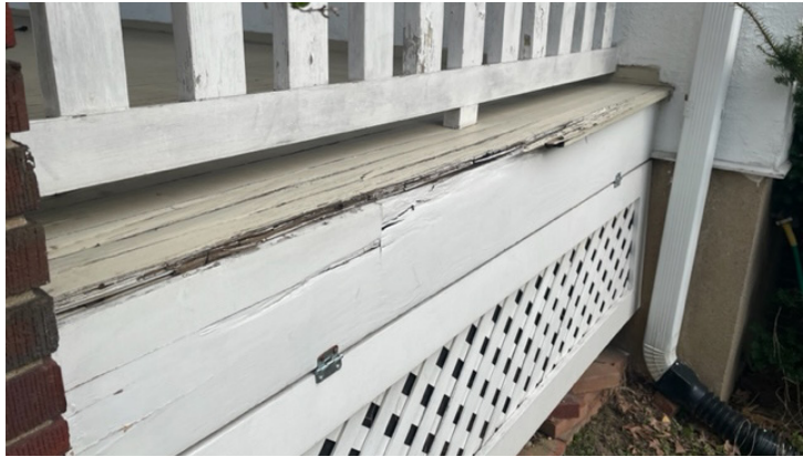
detail of damage at south end
