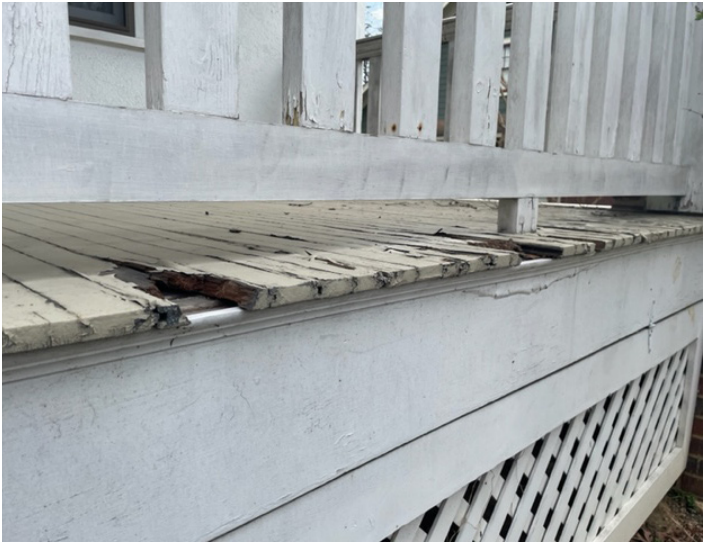
detail of damage at west edge (front)
