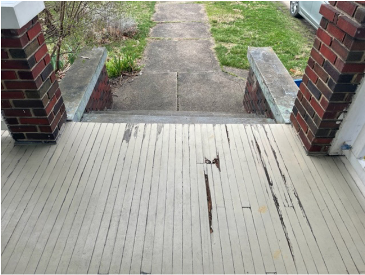
detail of damage at west edge / stair
