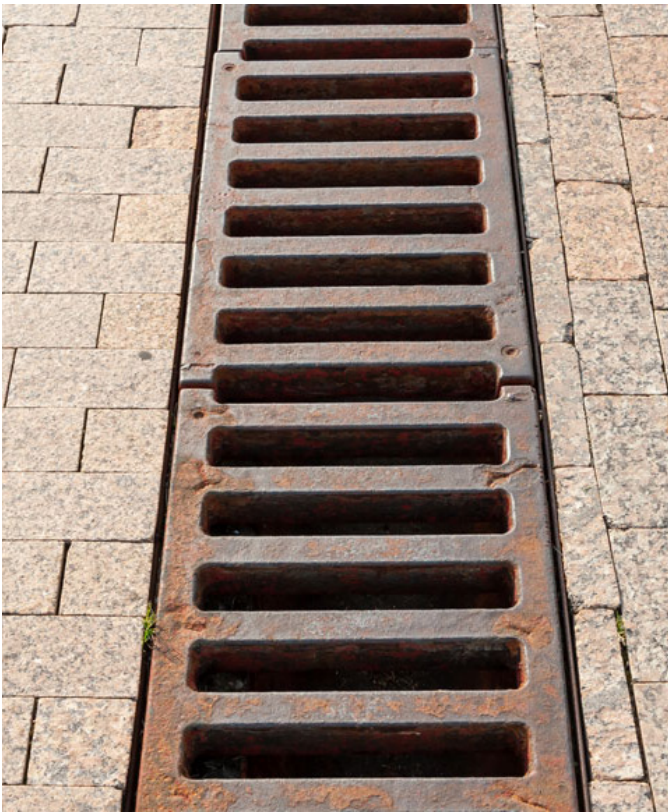
trench drain example
