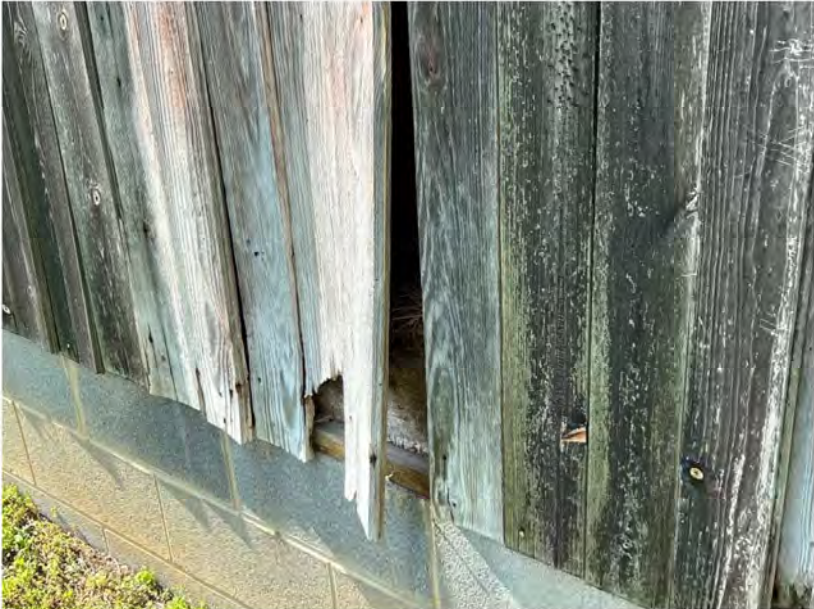
Figure 3. South Elevation: Peeling and Deteriorating Siding
