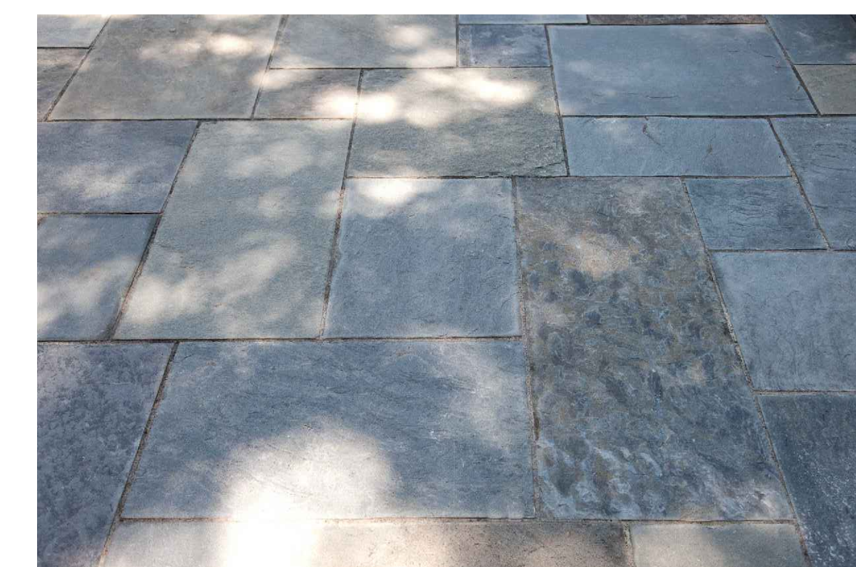
STONE POOL DECK, TERRACE AND WALKWAYS EXAMPLE (PENNSYLVANIA BLUESTONE W/NATURAL CLEFT & FULL RANGE COLOR)
