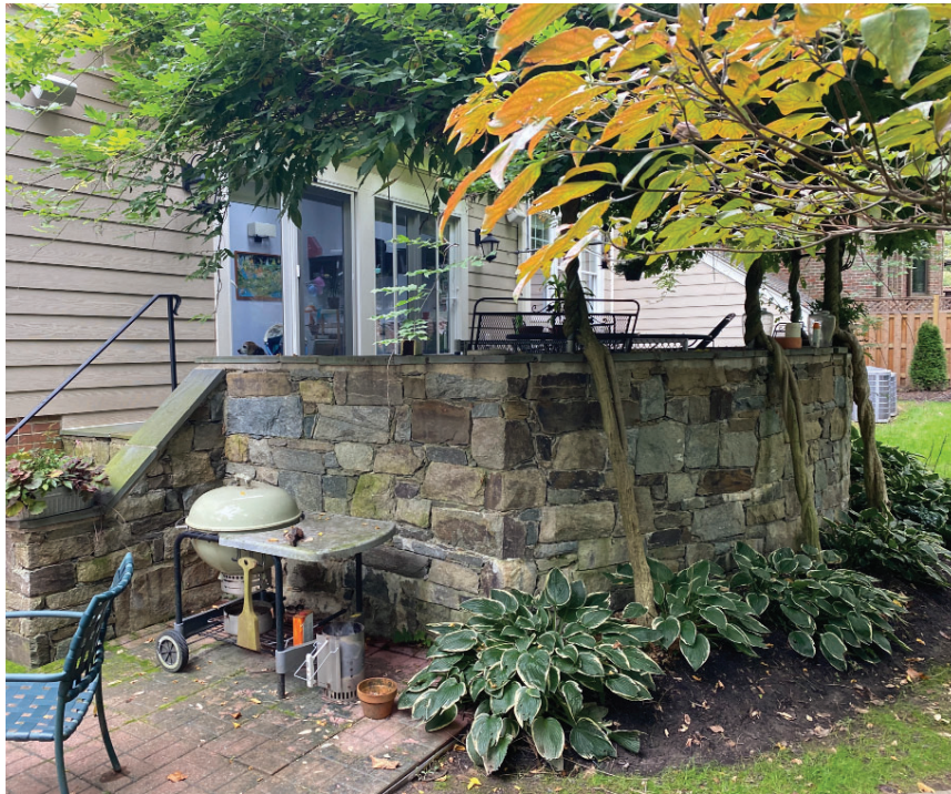
EXISTING MASONRY DECK AND SUNROOM EXTERIOR DOORS AS VIEWED FROM REAR YARD
