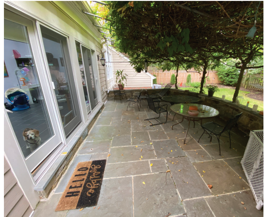
EXISTING MASONRY DECK SPACE AND SUNROOM EXTERIOR DOORS AS VIEWED FROM TOP OF DECK STEPS
