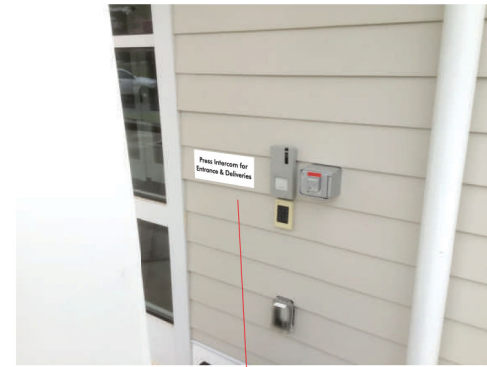
Close Up View - As Installed
