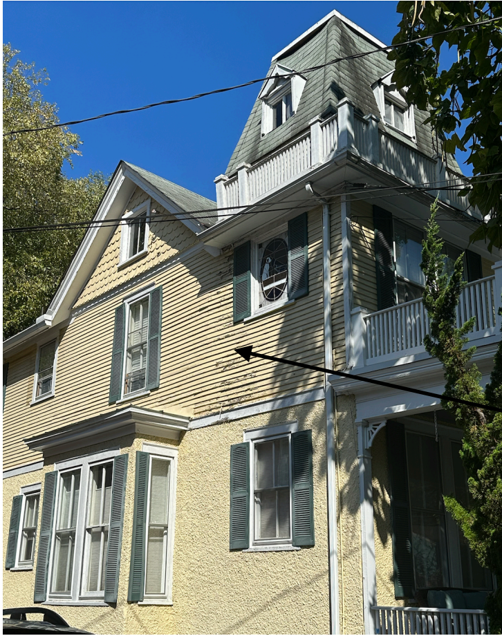
You can see the water damage on the house from the roof.
