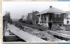
ON THE RIGHT SIDE IS THE SECOND STATION BUILDING UNDER CONSTRUCTION IN 1928. THE FIRST STATION BUILDING, ON THE LEFT SIDE, WAS BUILT IN 1887. (Courtesy: John K. King Collection and John S. Collier)
