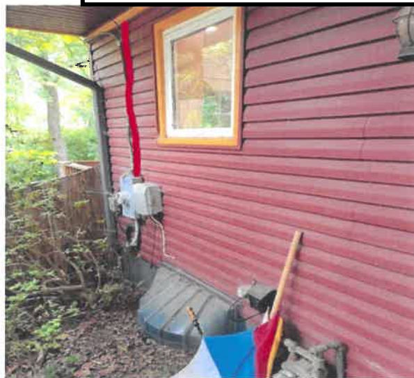
Utility Side Example After Installation
