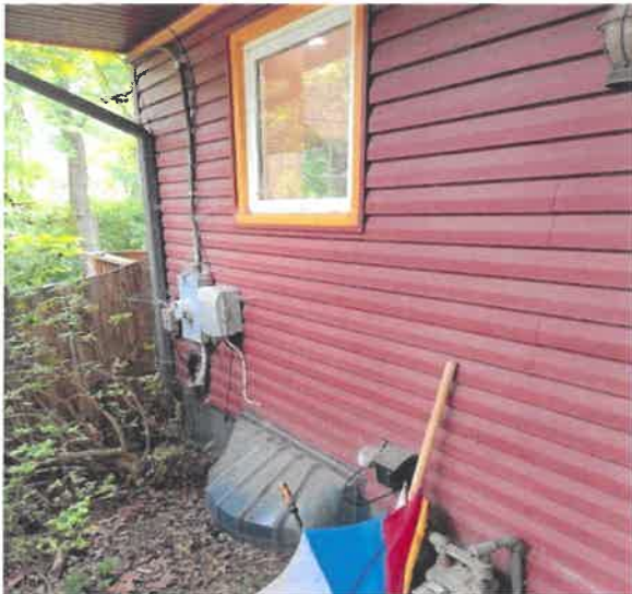
Utility Side Before Installation
