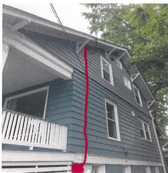
Utility Side Example After Installation
