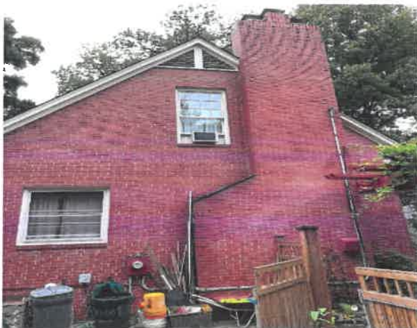
Utility Side Before Installation
