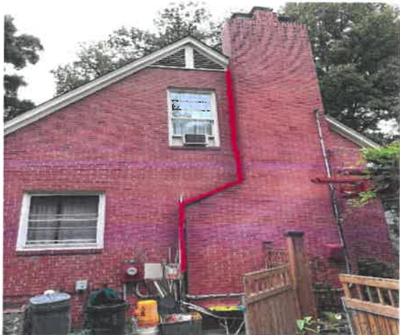
Utility Side Example After Installation
