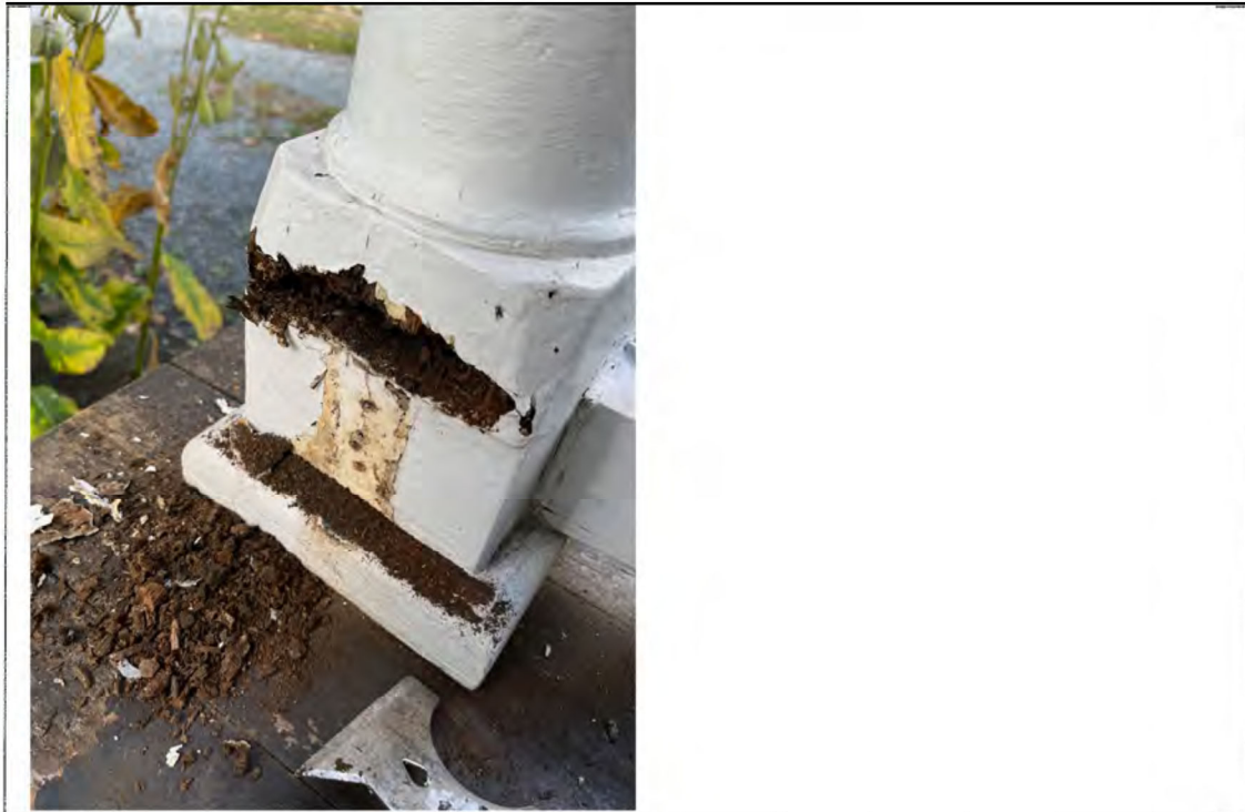
Detail: "soggy bottom rot" on porch post
