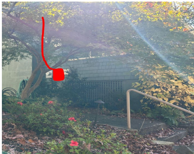
Utility Side Example After Installation
