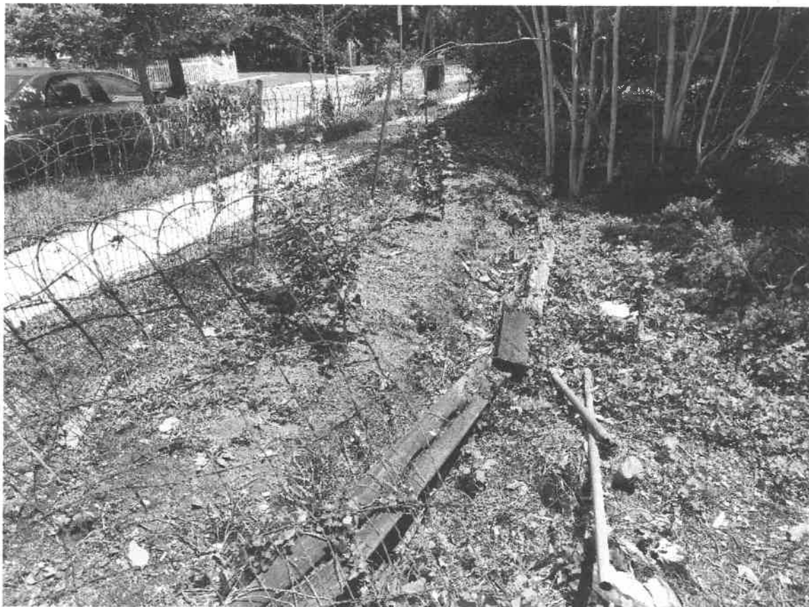
Failing retaining wall and fence, photo taken from 3806 Baltimore St driveway
