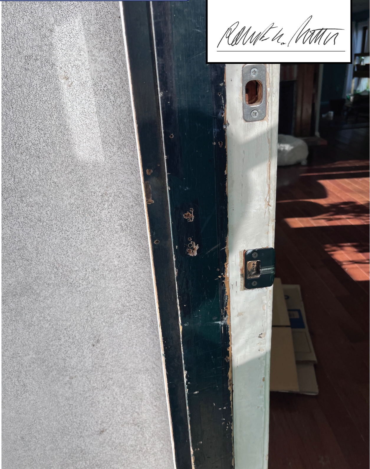
Weathering of wooden frame for exterior door to entryway
