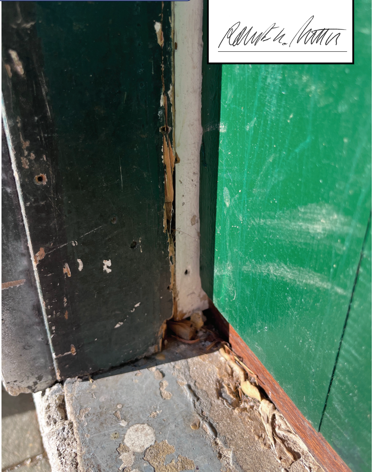
Close up of damage to wood and cement threshold of exterior door to entryway
