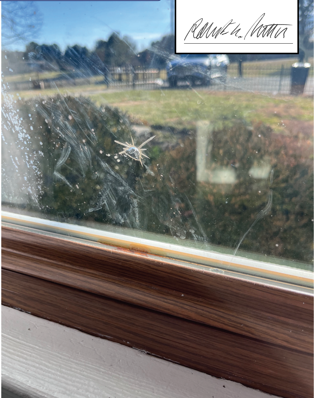
Damage to glass on second window in living room
