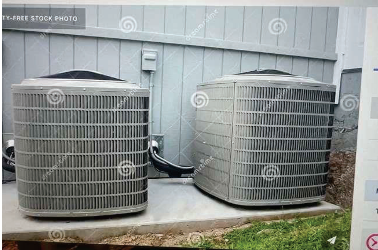
Sample photo of the AC units
