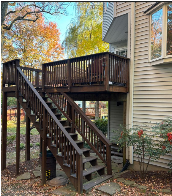
Side View of existing Pressure treated wood deck and stairs- to be demo'ed. New P.T screen porch, deck, landing and stairs will be build in
