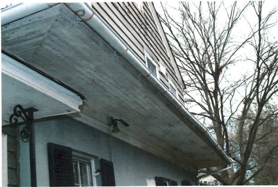
Additional Photo 3. 02/19/20. Side (east). Exterior. Roof. Project area. Gutter at bottom of roof is in need of replacement.
