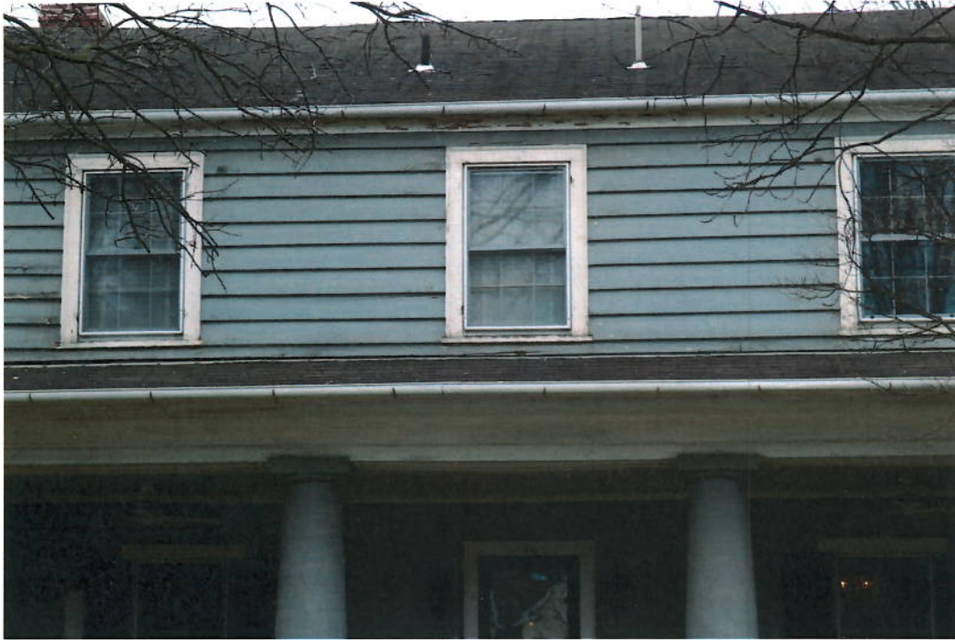
Additional Photo 1. 02/19/20. Front (north) elevation. Exterior. Roof. Project area. Roof on top of the house and on top of the eave is deteriorated and in need of replacement.
