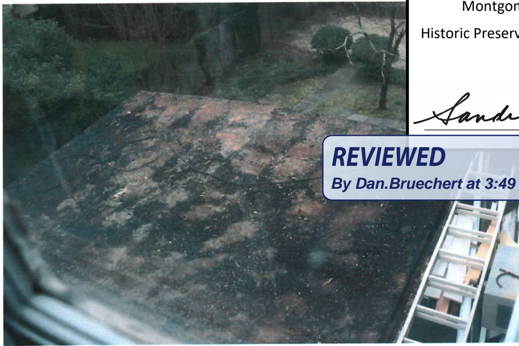
Additional Photo 4. 02/19/20. Back. Exterior. Roof. Project area. Flat roof over 1 st floor family room is deteriorated and in need of replacement. Gutter at bottom of roof is in need of replacement.
