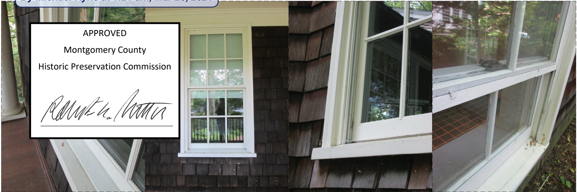
EXISTING WINDOW PHOTOS SHOWING PLASTIC JAMB LINERS, SPACER BARS AT SDL WINDOWS AND MODERN SASH LOCK HARDWARE
