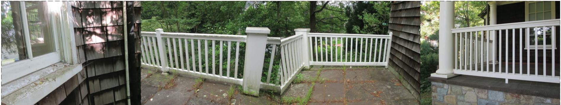
PHOTOS OF CURRENT 2ND FLOOR DECK RAILING WITH EXPOSED FASTENERS AS COMPARED TO MORE TRADITIONAL 1ST FLOOR PORCH RAILING
