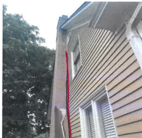
Utility Side Example After Install
