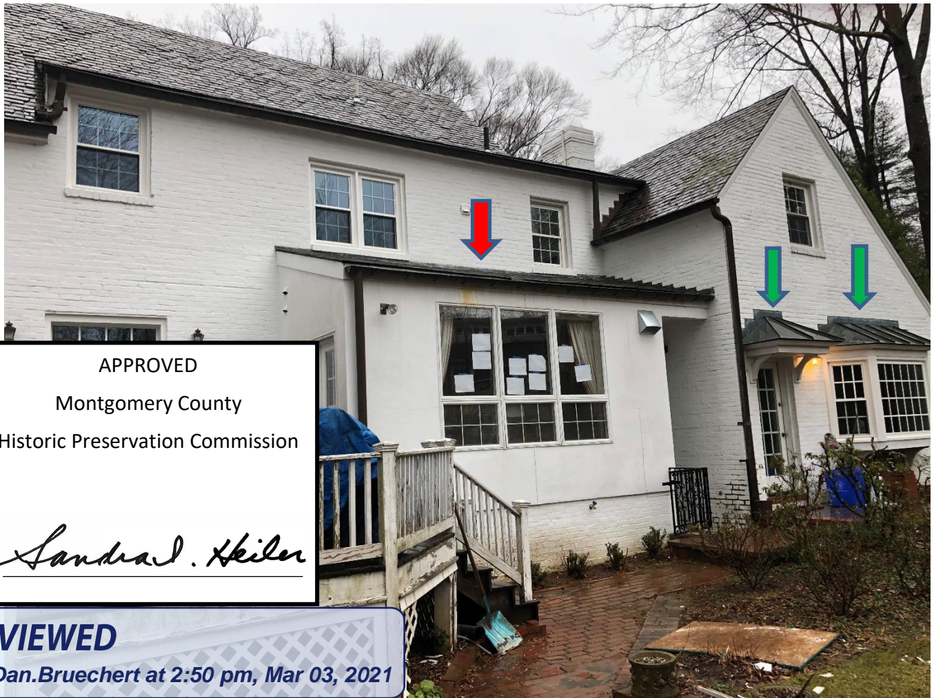
Figure 5: Slate roof on kitchen bump-out (red arrow). Current copper roofing (green arrows)
