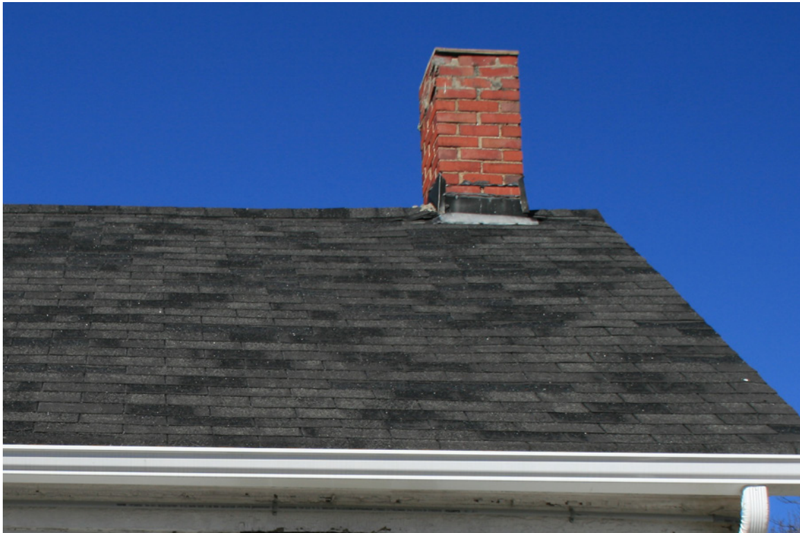
Photo 12 Close up view of existing 3-Tab shingles to be replaced like-in-kind. Photo by Ward Bucher | March 01, 2020
