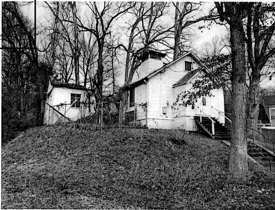
Photo No. 8: View of damaged structure looking Northwest
