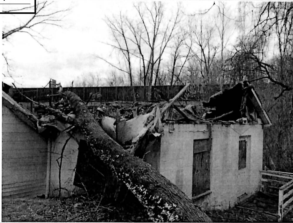
Photo No. 4: Rear (West) elevation view of damaged structure
