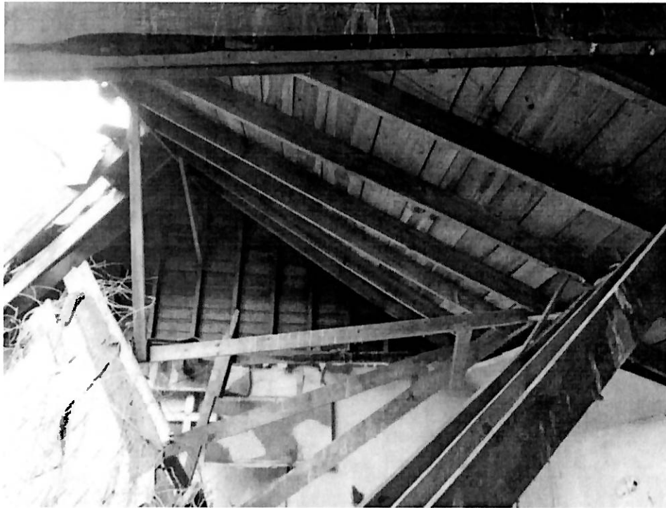
Photo No. 13: View collapsed roof framing along the west end of the structure. Note that wall and roof framing consists of 1" thick wood boards of various widths attached to solid sawn rafters or studs.
