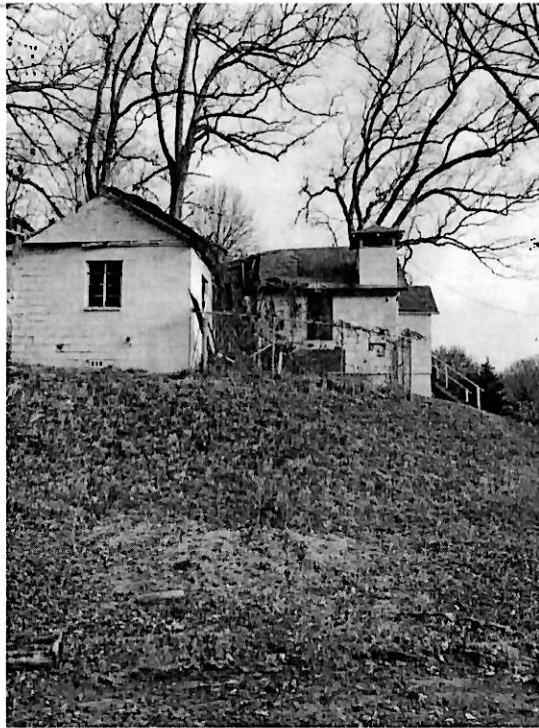
Photo No. 6: Left Side (South) elevation view of damaged structure Detail: _____
