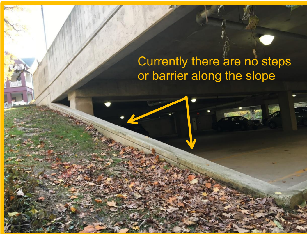
View of the slope from the covered garage to the parking deck above.
