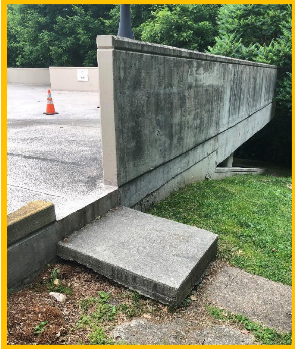
View of the existing pedestrian opening on the upper parking deck of the garage.
