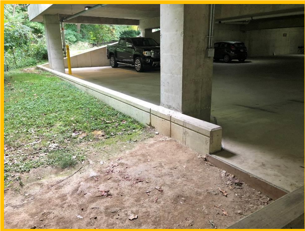
View of the back of the lower level of the garage showing the existing pedestrian opening into the garage where the walkway will be constructed. The slope where the stairs will be constructed is at the upper left side of the photo.
