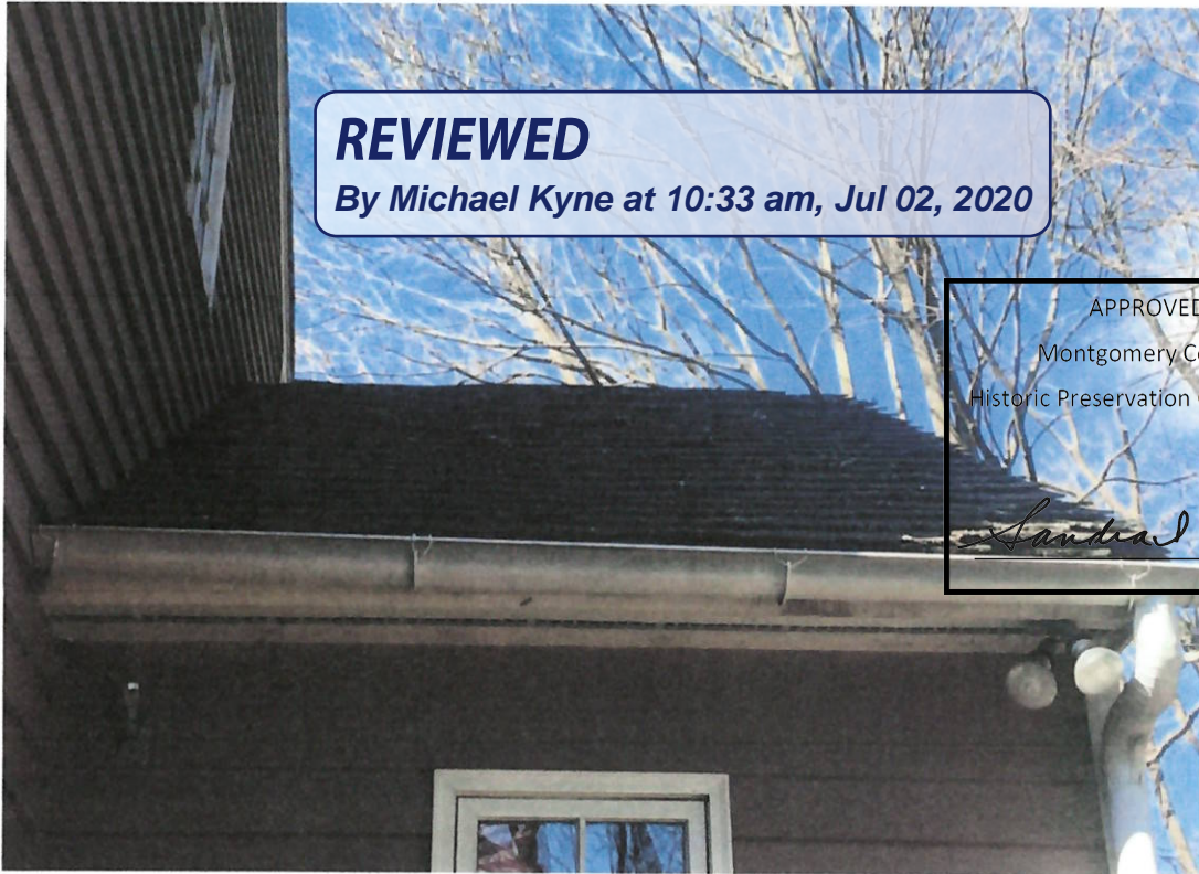
Damaged Shingles – Damaged Gutter 1
