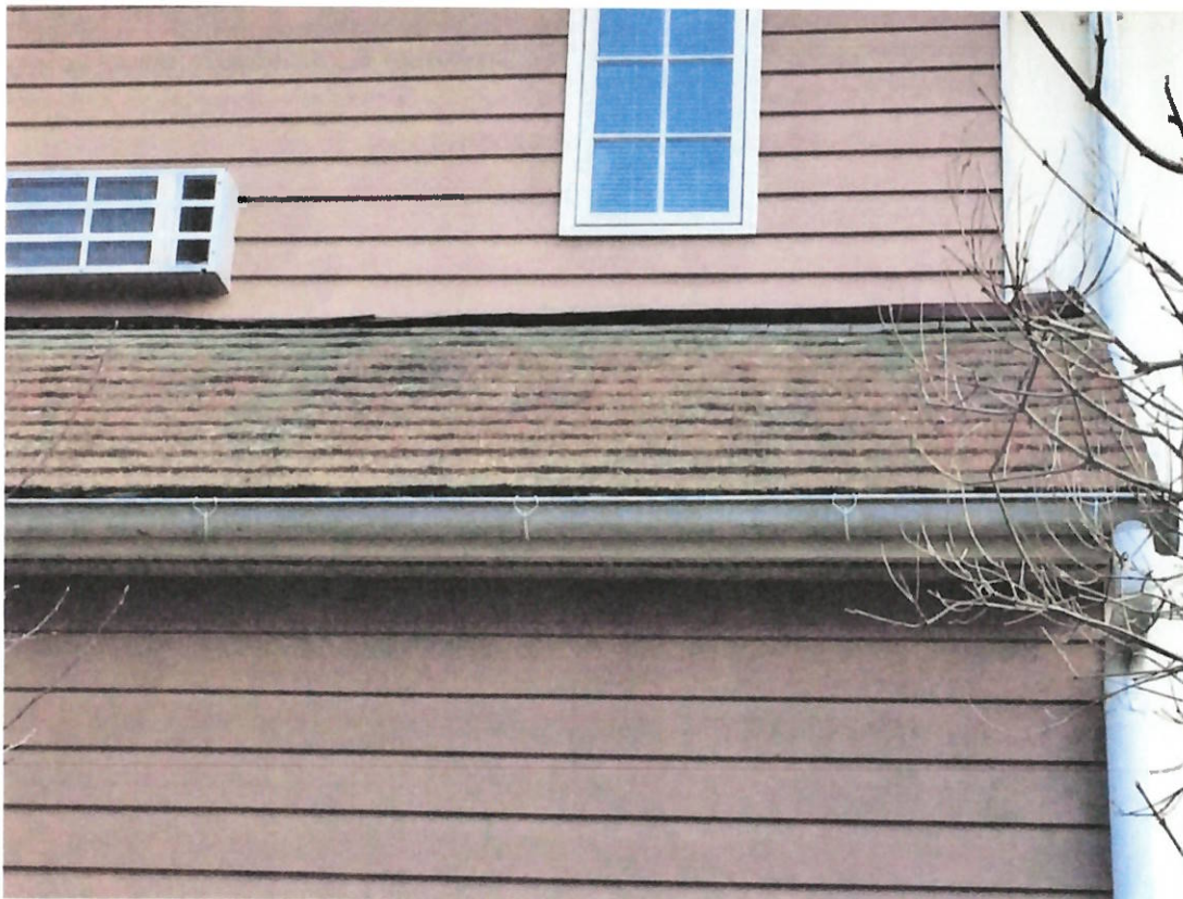
Damaged Flashing – Moss on Shingles
