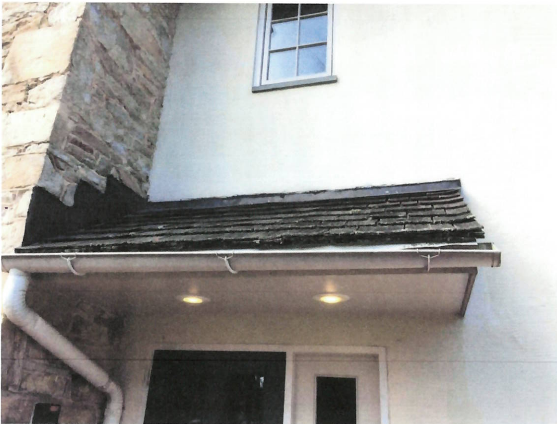
Damaged Shingles – Damaged Gutter 2
