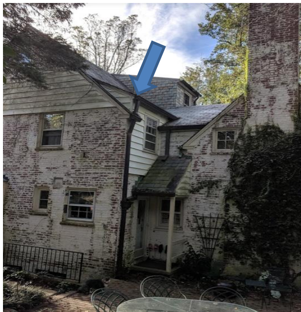
Detail: East side of house, showing location of low sloping roof section proposed for renovation
