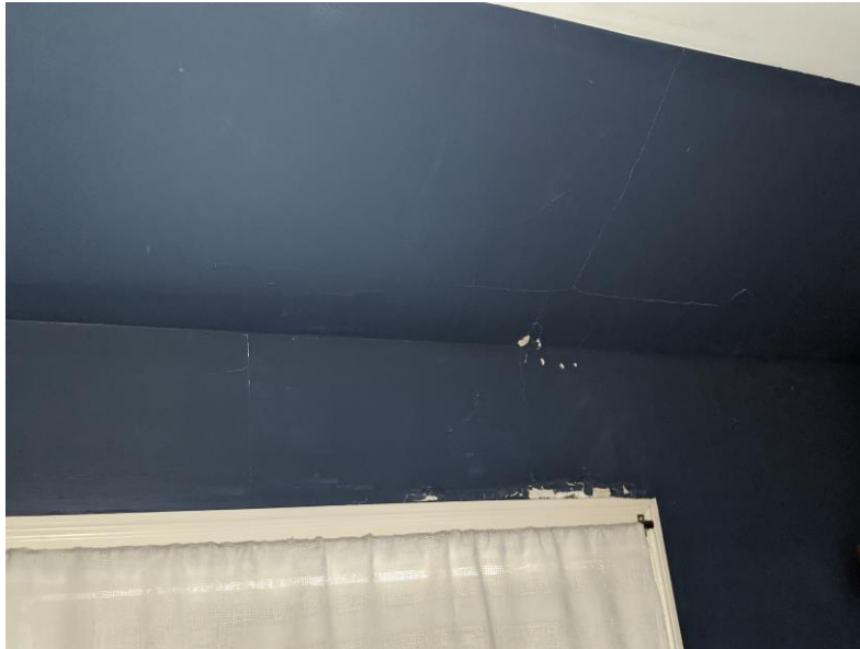
Figure 3. Water damage below low-sloping shed dormer roof
