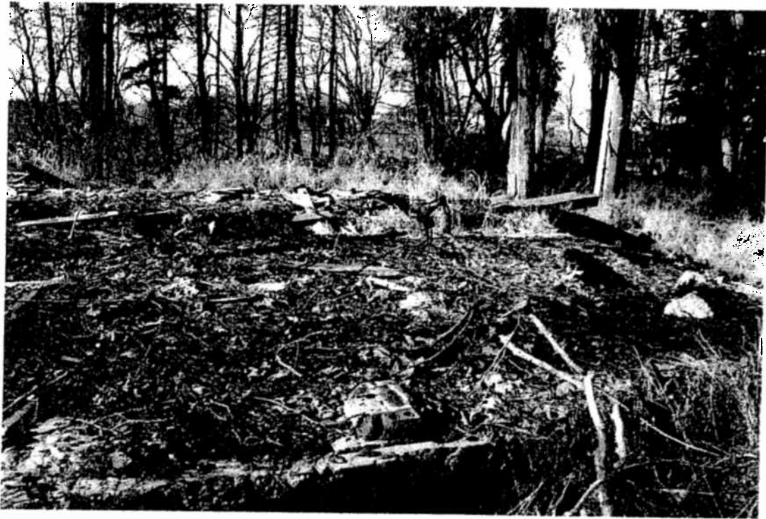
Figure 4. Concrete slab foundation ruins, December 2011.
