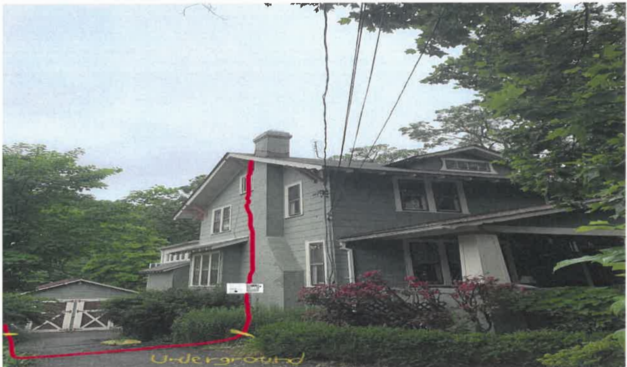
Equipment Location and Conduit, After Installation
