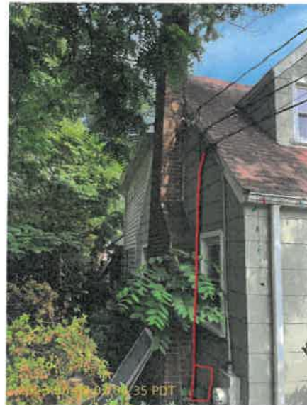
Utility Side After Installation
