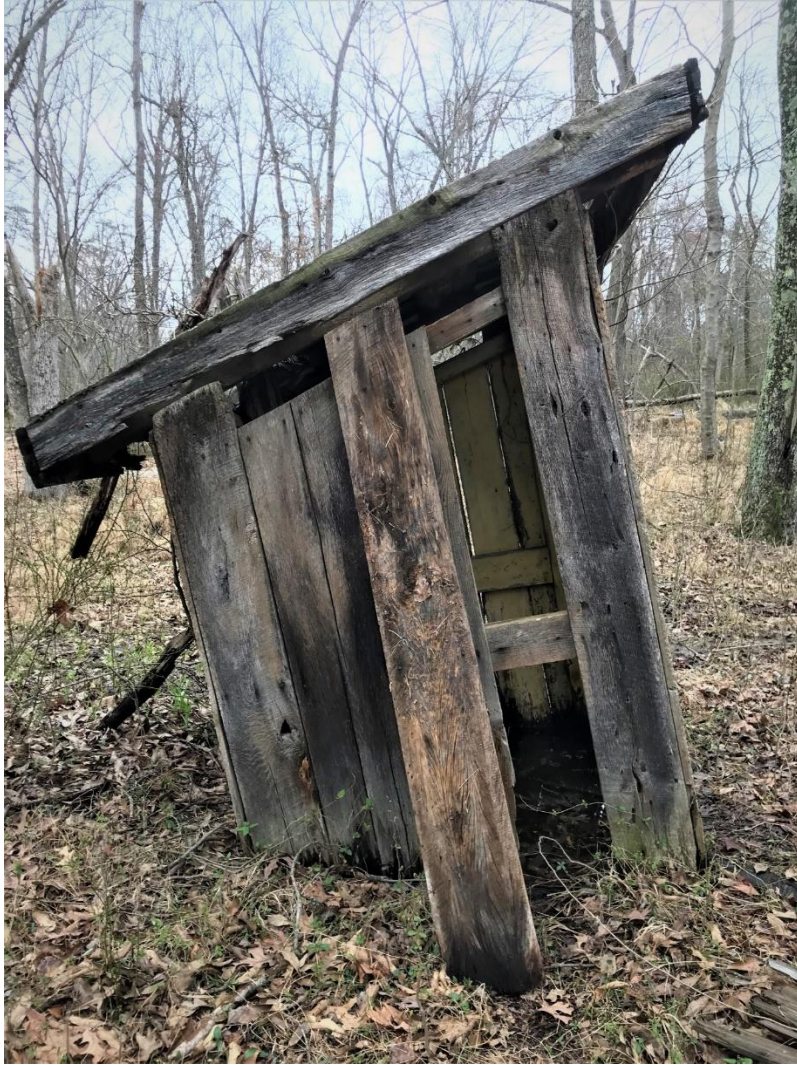
Side view: tilting and missing sideboards – note the decayed and rotten condition of the sideboards.
