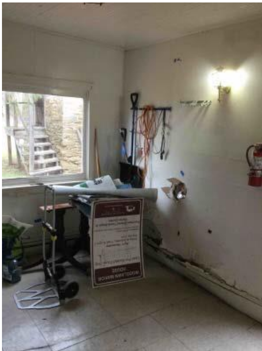
Interior of mudroom showing east wall (right) with separation of wall at foundation.
