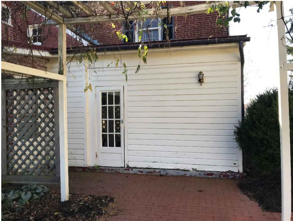
East elevation of mudroom. Note deterioration at sill. Wall is nearly detached. Also note door is no longer plumb. The good condition of the siding belies the deteriorated structural condition of the wall.
