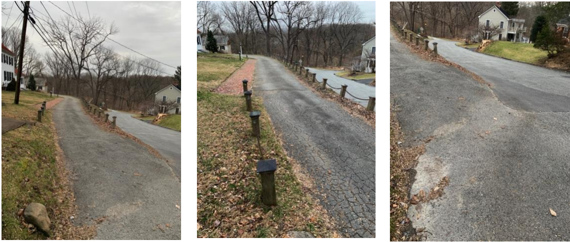
Figure A-1: Race Street Conditions (Note: Significant Cracking and Uneven Pavement/Asphalt of Race Street)
