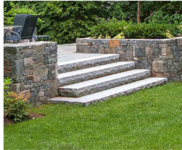
STONE STEPS, HIDDEN MORTAR WALL
