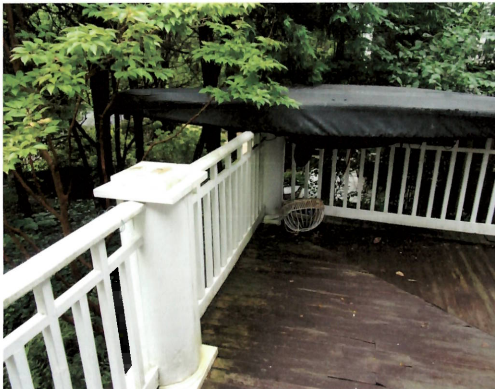
Two Rail Columns to be replaced.
