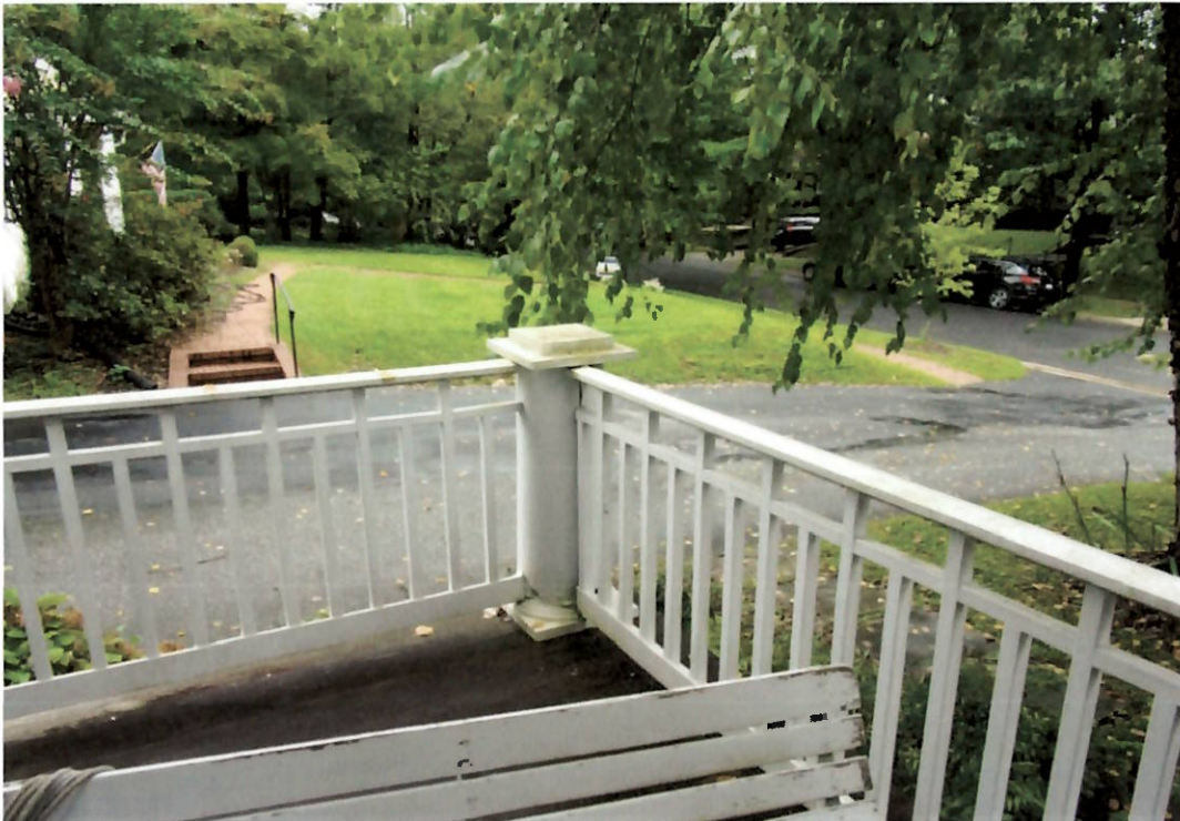
One of three rail columns to be replaced (rail to right also needs replacing).
