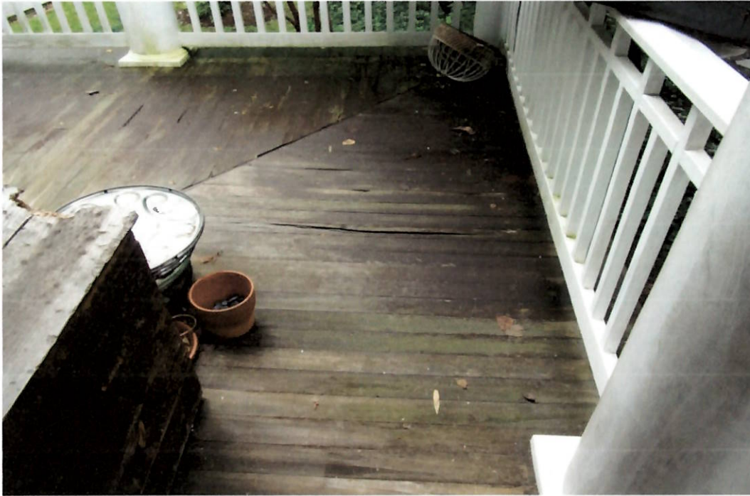
Area of damaged floor.
