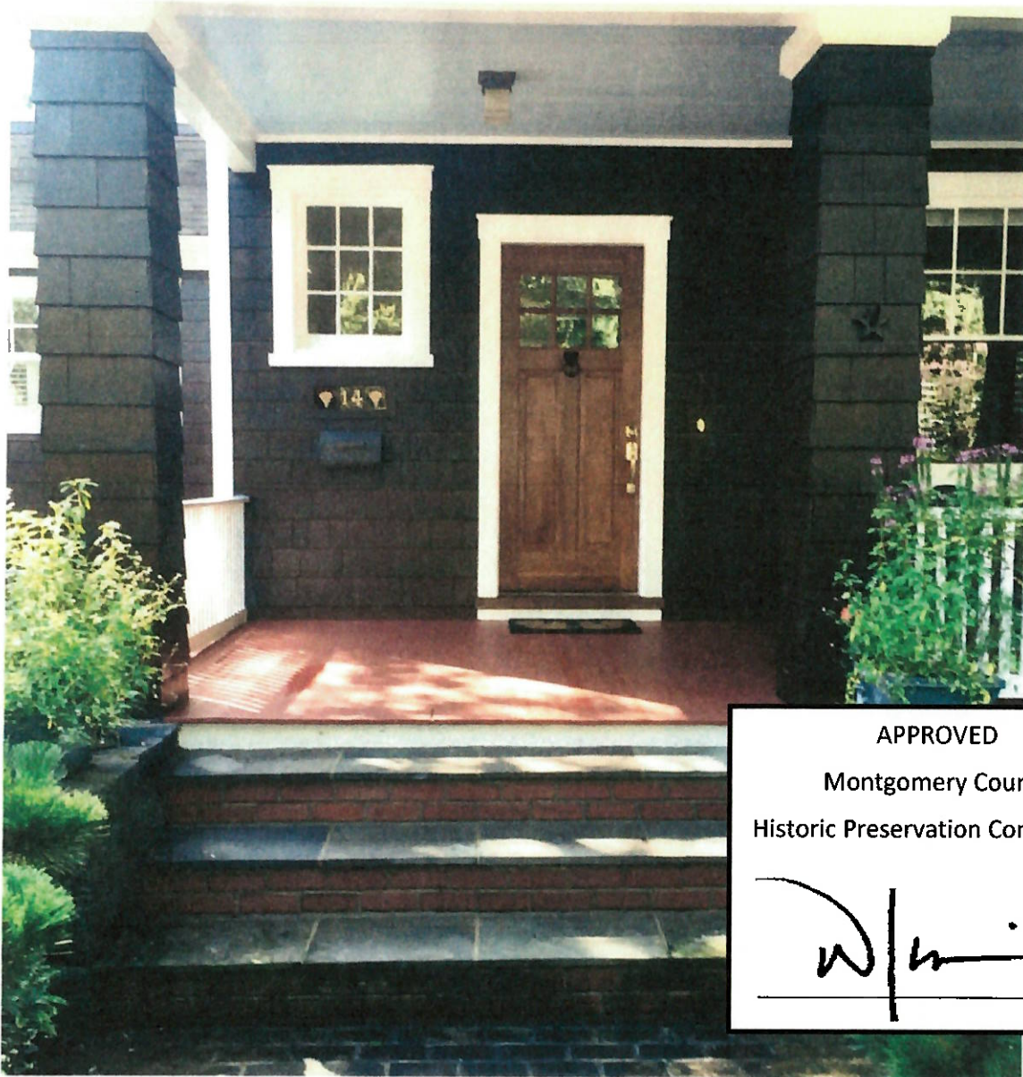
Existing front stairs without railings.
