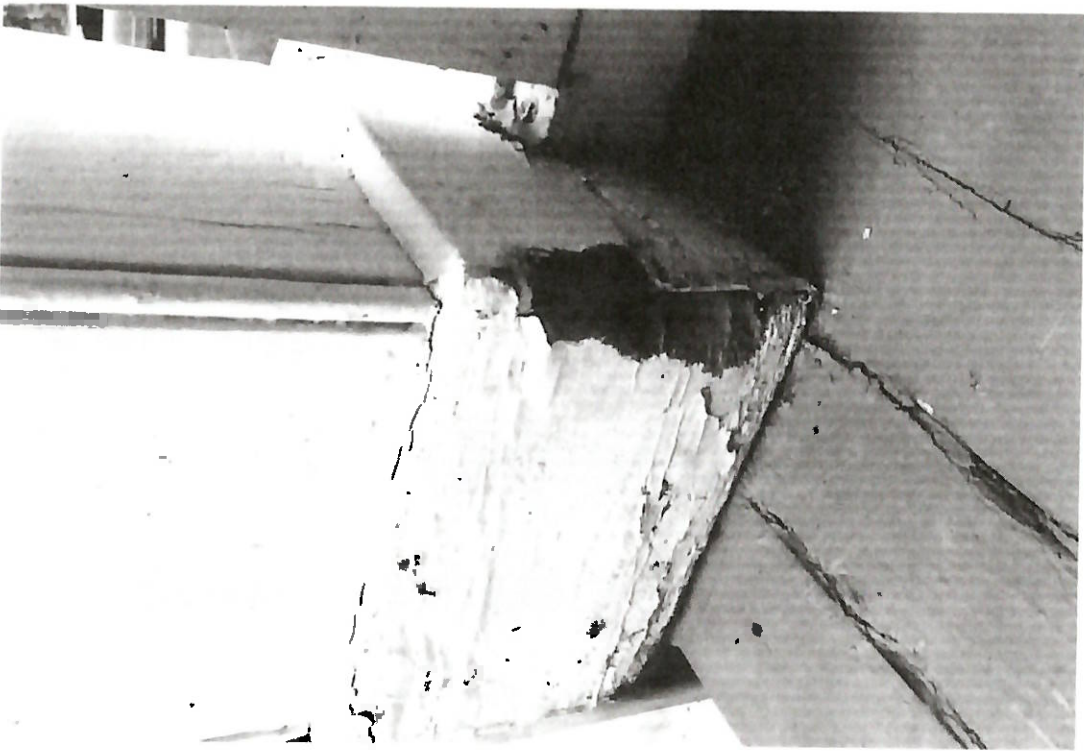
WOOD STAIR, PAILING, POSTS (TO BE RESTORED, REPAIRED, REPLACED)
