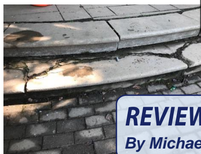
Crumbling stairs in the center of the patio leading to the lawn
