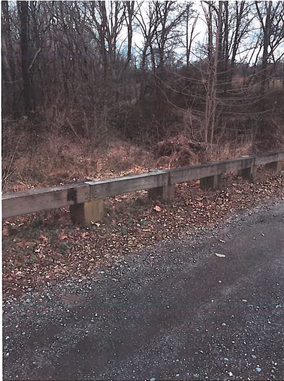
Photo of extant guardrail at Black Hills Regional Park as example of what is proposed at this site.
