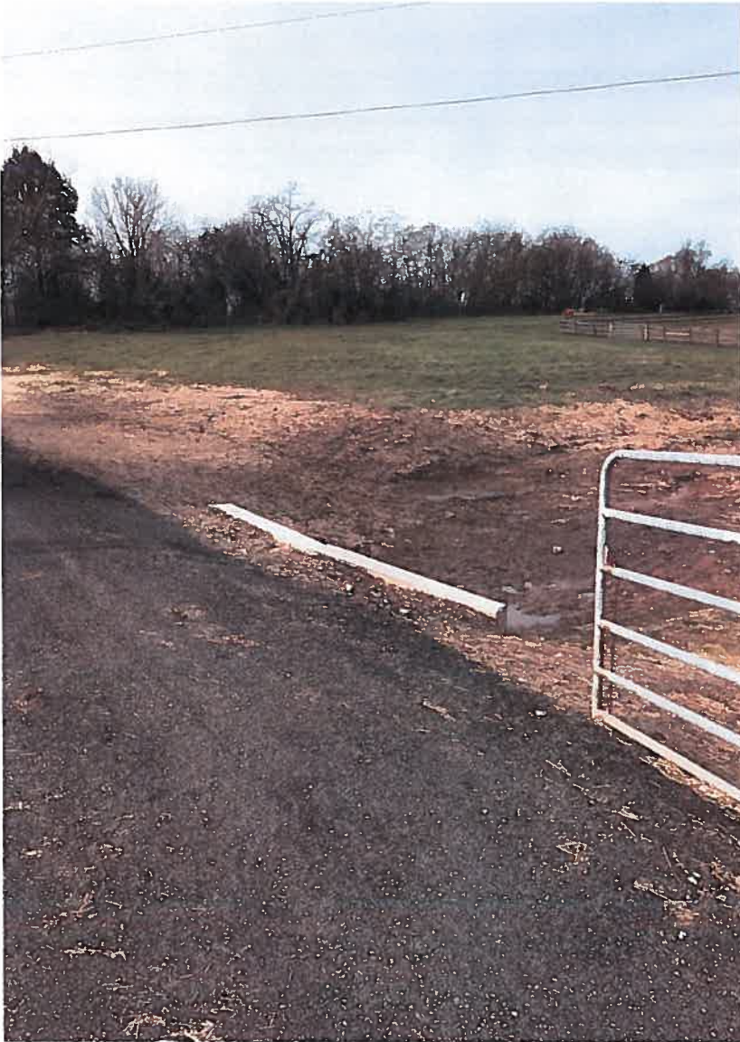
North side of the culvert (open horse gate on right). Millings to be removed and grass restored following completion of construction work. House is located beyond the photo to the upper left-hand corner.
