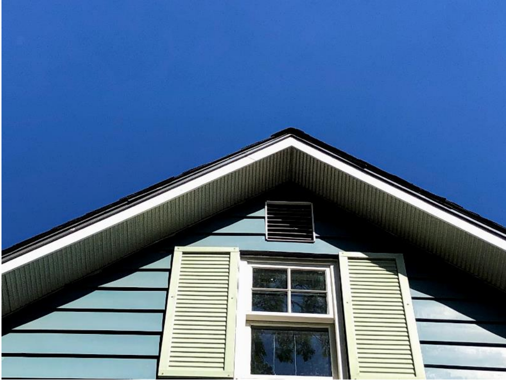
View of non-historic aluminum rake soffit
