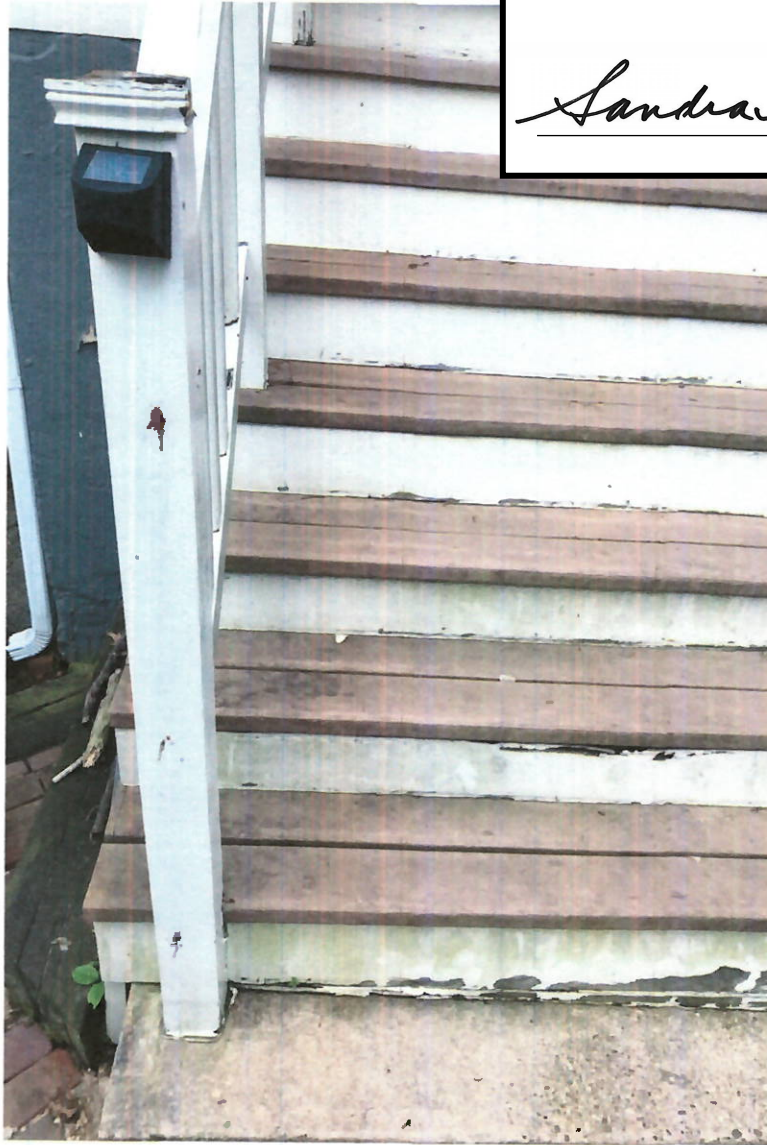
close-up to show composite material on steps - would be replaced with wood.
