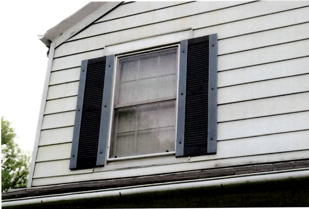
Photo 10. 08/05/19. Side (east) elevation. Project area. Left close-up showing aluminum siding to be removed; non-original shutters to be replaced and painted; aluminum gutters to be repaired.
