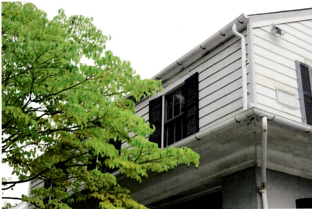
Photo 4. 08/05/19. Front (north) elevation. Project area. Right close-up showing aluminum siding to be removed; shutters to be restored and painted; wood porch ceiling, trim, and molding to be repaired and painted; stucco to be repaired and painted; aluminum gutters and downspouts to be repaired.
