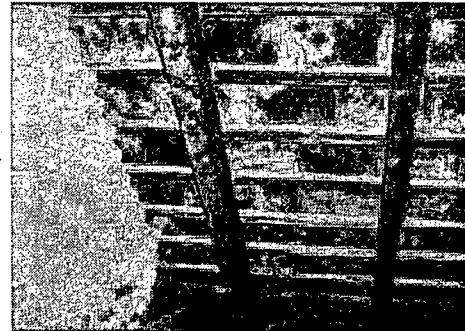
View of these slates laid on open sheathing shows that delamination and flaking are just as bad or worse on the underside of slates as on the exposed surface. This is why most slates cannot be flipped over for reuse. Photo: Jeffrey S. Levine.
